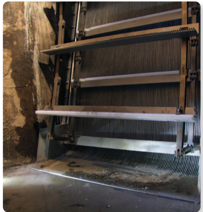
Curved Bar Rack at Channel Bottom
